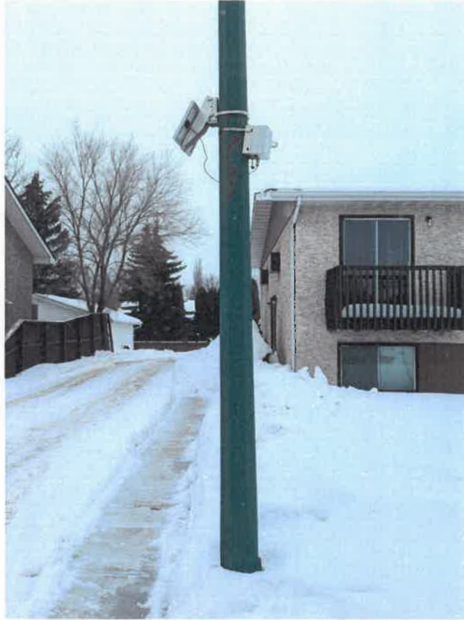
Traffic Counter Mounted on a Streetlight
